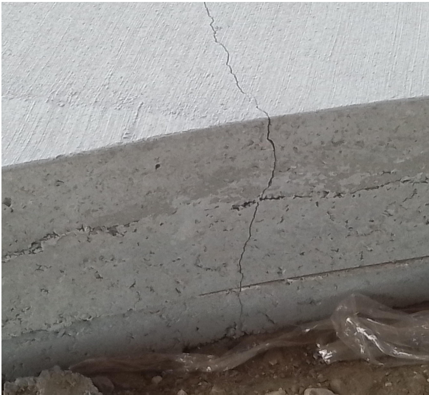
Concrete slab cracking. Image courtesy of APEX (09.08.23)
