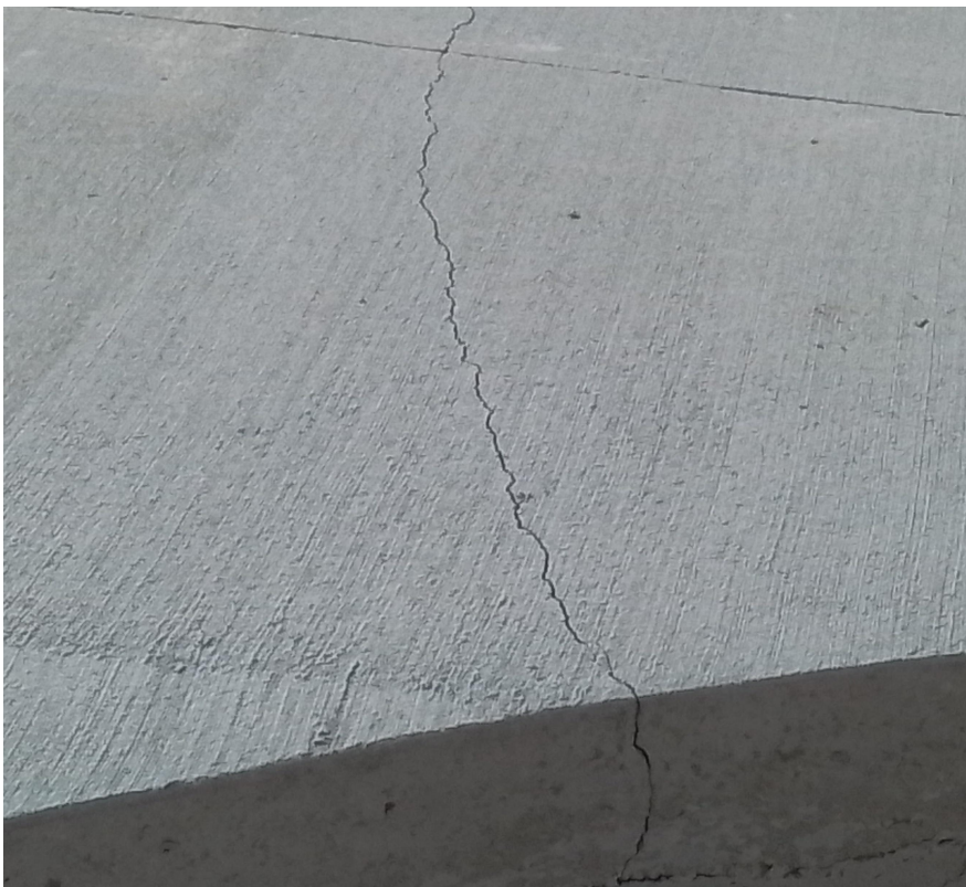
Concrete slab cracking. Image courtesy of APEX (09.08.23)
