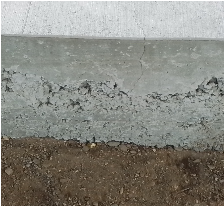
Concrete slab cracking. Image courtesy of APEX (09.08.23)
