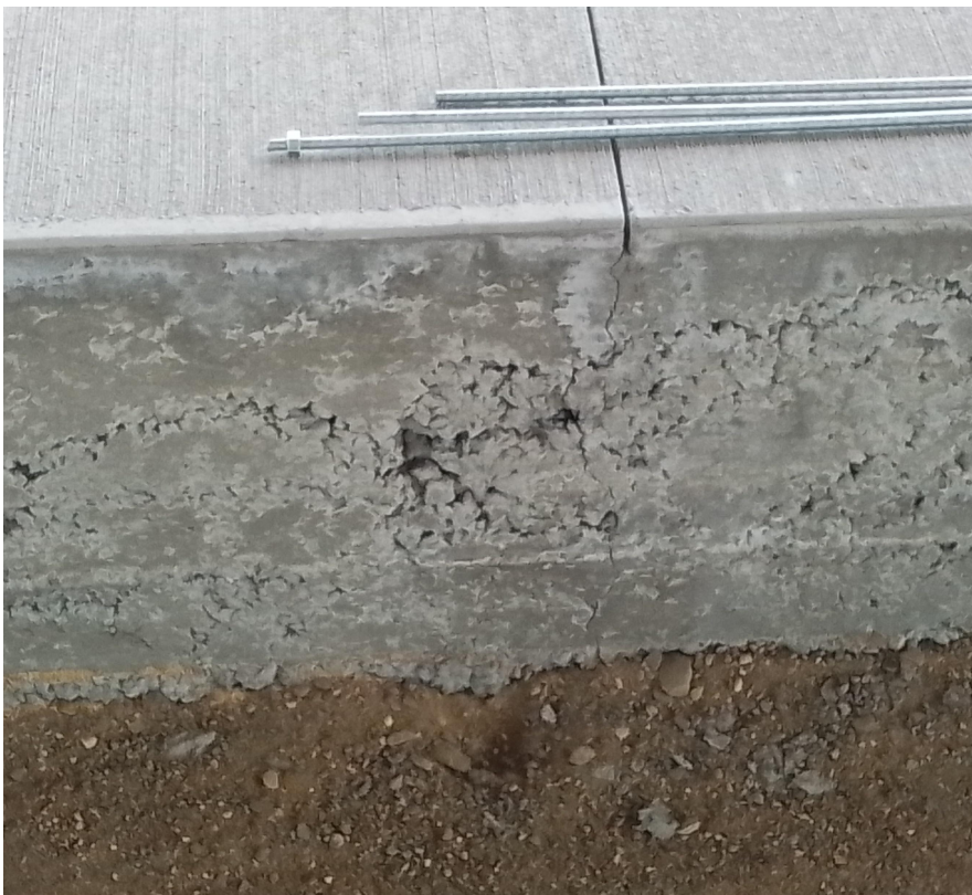
Concrete slab cracking. Image courtesy of APEX (09.08.23)
